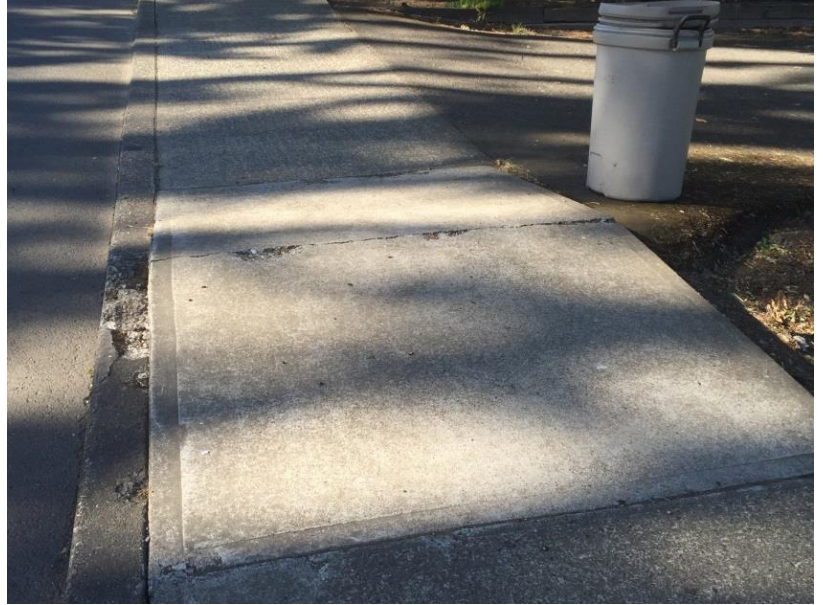
Sidewalk on east side of Main Street (OR47) with cracks and buckling
