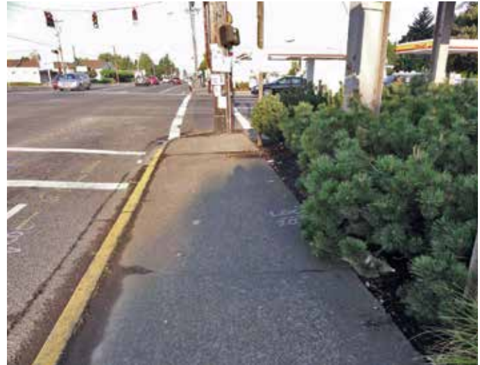
A non-compliant ADA ramp at SE Division Street and SE 182nd Avenue.
