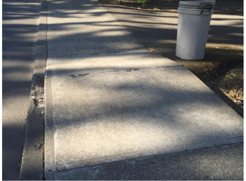
Sidewalk on east side of Main Street (OR47) with cracks and buckling
