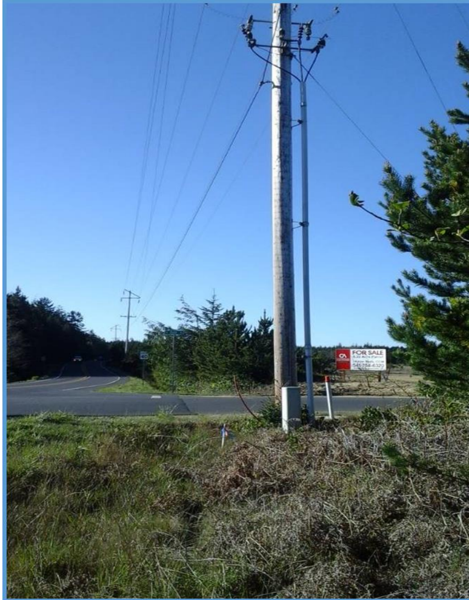
Image 3.1: Three Phase Power Running Along East Edge of Site
