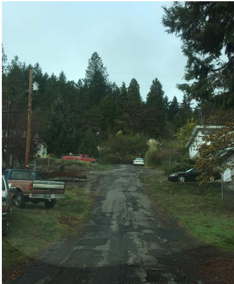
Example of roadway in need of repaving
