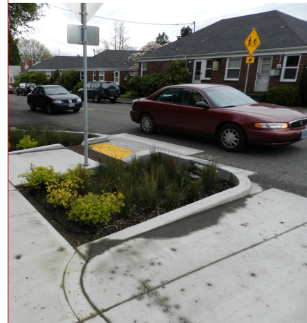
This is representative of the treatment that may be included at the intersection corners to capture stormwater runoff before it can reach the storm sewers.
