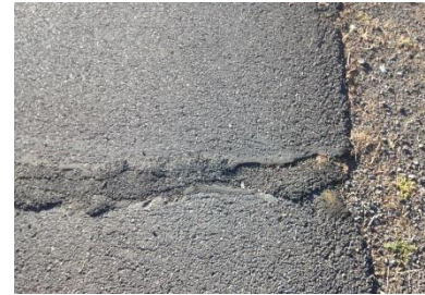
Patched Crack on OC&E Trail
