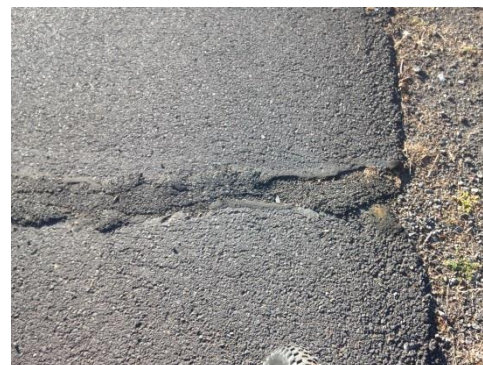
Crack in trail pavement
